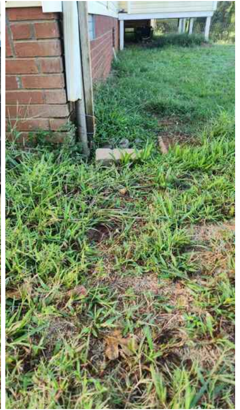
Back corner hole at downspout and slopes to crawlspace access.
