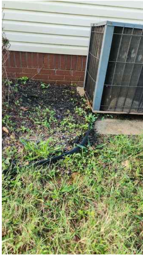
Water runs toward AC unit. Could run under house.
