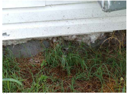
Next to ac unit
