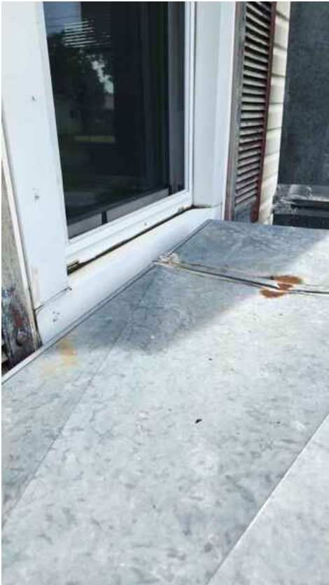
Bottom window trim slopes toward window
