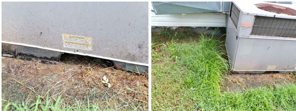
Can't tell where the water is coming out from No condensate pipe
