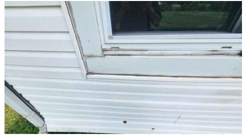
Back patio window needs caulk touch up
