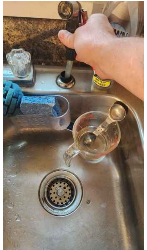
Sprayer wand ring in broken or loose
