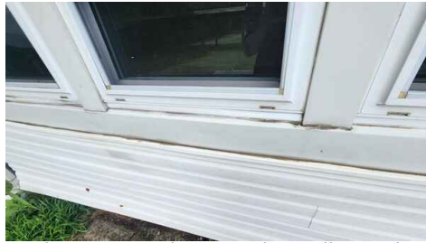
Back patio window needs caulk touch up
